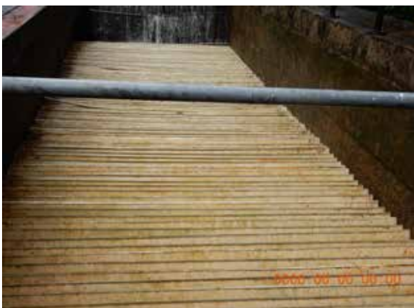
Figure 5 - Plate settler sedimentation tank after 10 years
